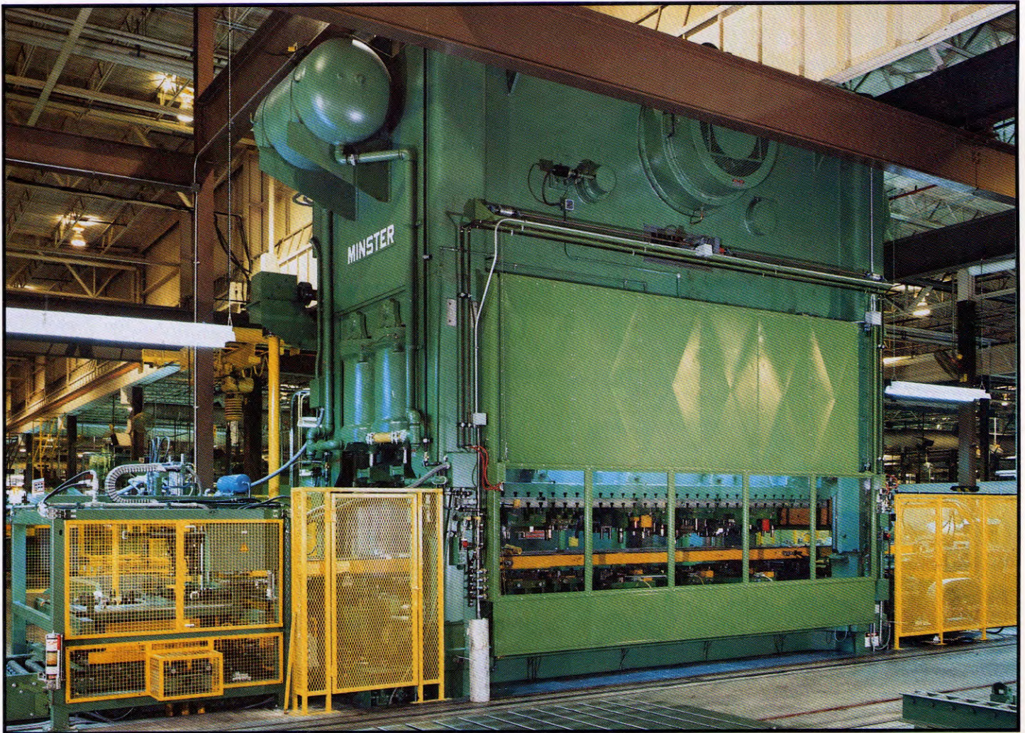
This new press/transfer system at Steelcase Inc. provides increased production speed and flexibility.
